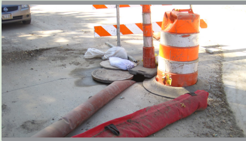
Sanitary Sewer Overflow or Dry-Weather CSO event
