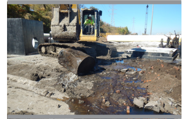
Leaking UST found during South Interceptor Force Main construction
