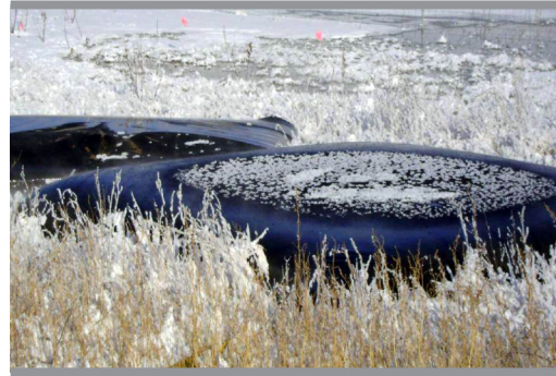
Erosion control at the discharge point with filter bags, jurisdictional wetlands in background
