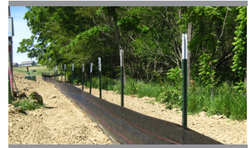
Construction "disturbed area" with silt fence properly installed and in good condition
